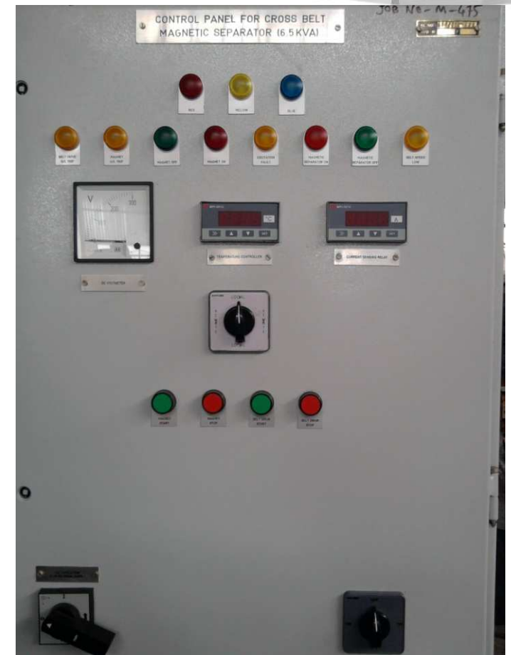
CBMS Control Panel for Vicat Sagar
