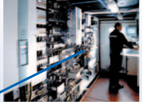
Air-conditioned electric compartment
