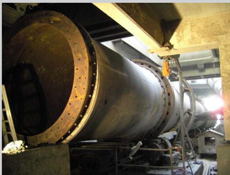
View on kiln drive system
