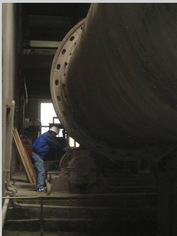
View on roller station 1
