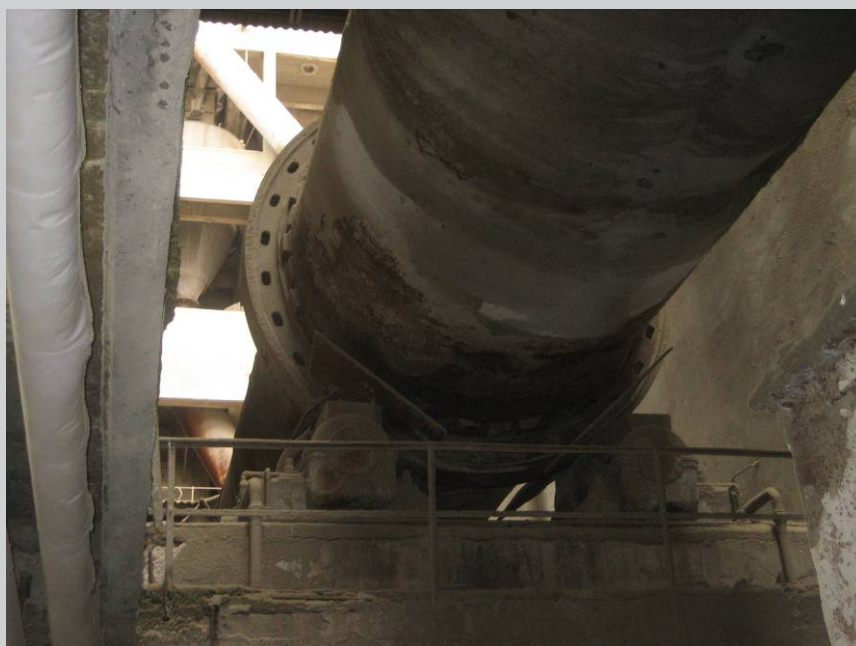
View on roller station 2
