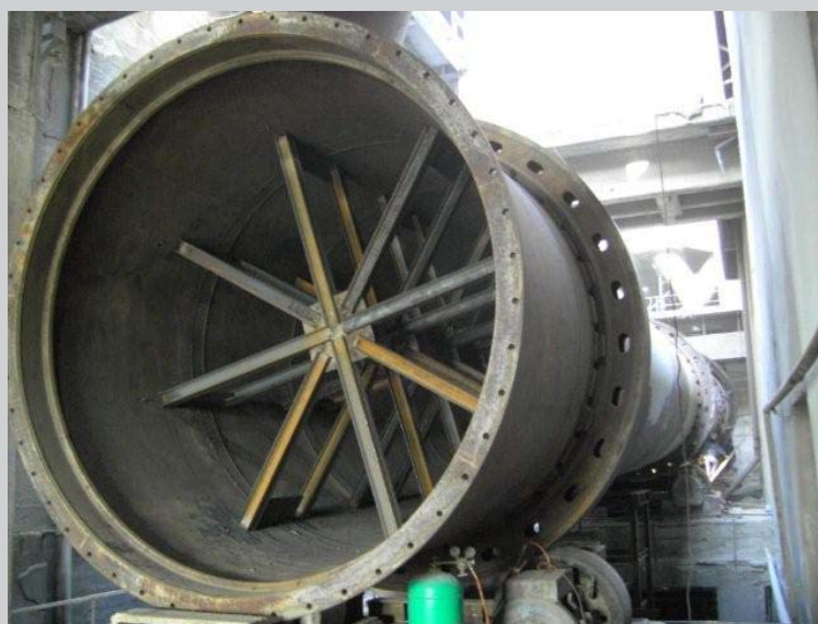
View on kiln outlet
