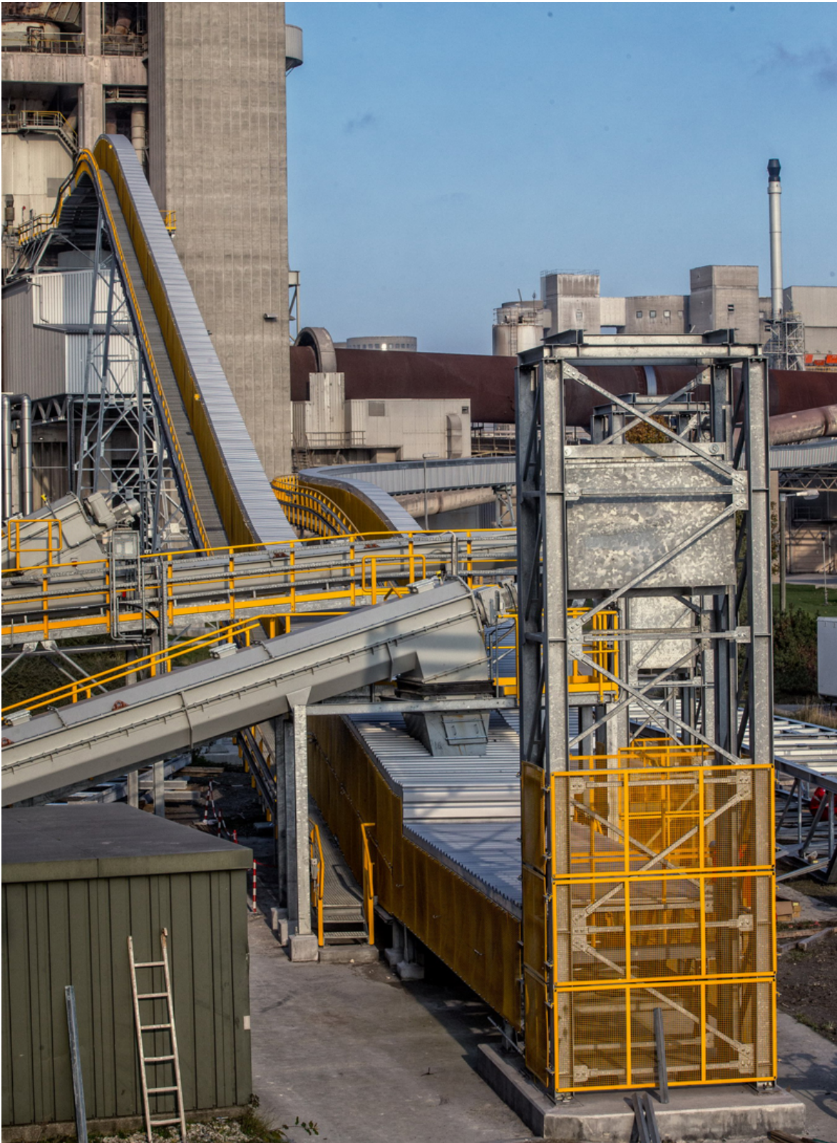
Fig. 2: The feeding station of the Pipe Conveyor to the calciner: at this regard, a take-up device has been installed at the rear.
