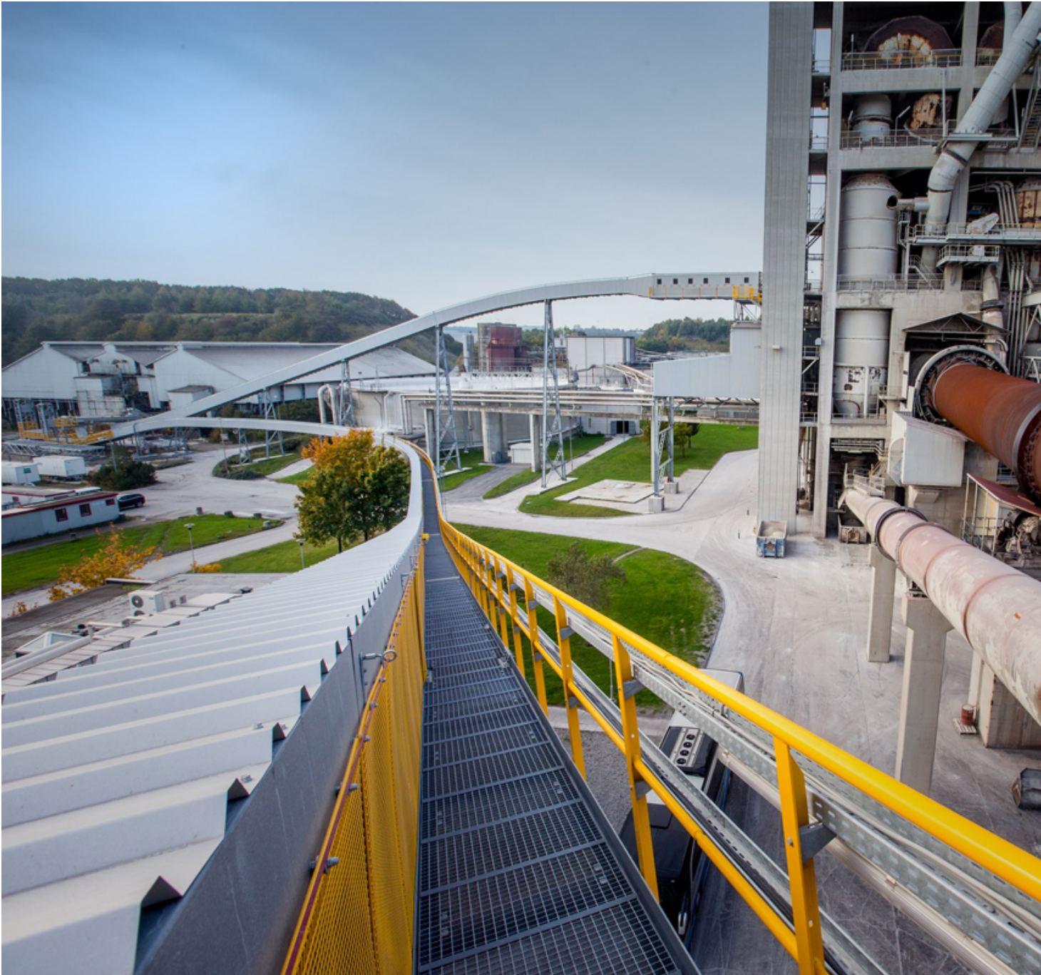
Fig. 3: The two Pipe Conveyors: BEUMER Group realises different system solutions for the various bulk materials.
