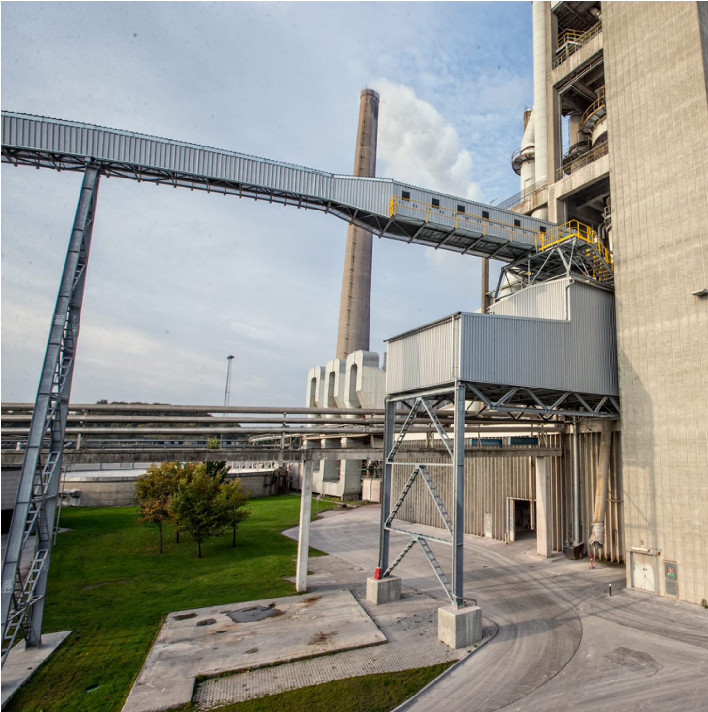
Fig. 5: The penthouse is underneath the discharge station of the Pipe Conveyor of the calciner. The intermediate hopper with the activator and the two double discharge screw conveyors are positioned here.
