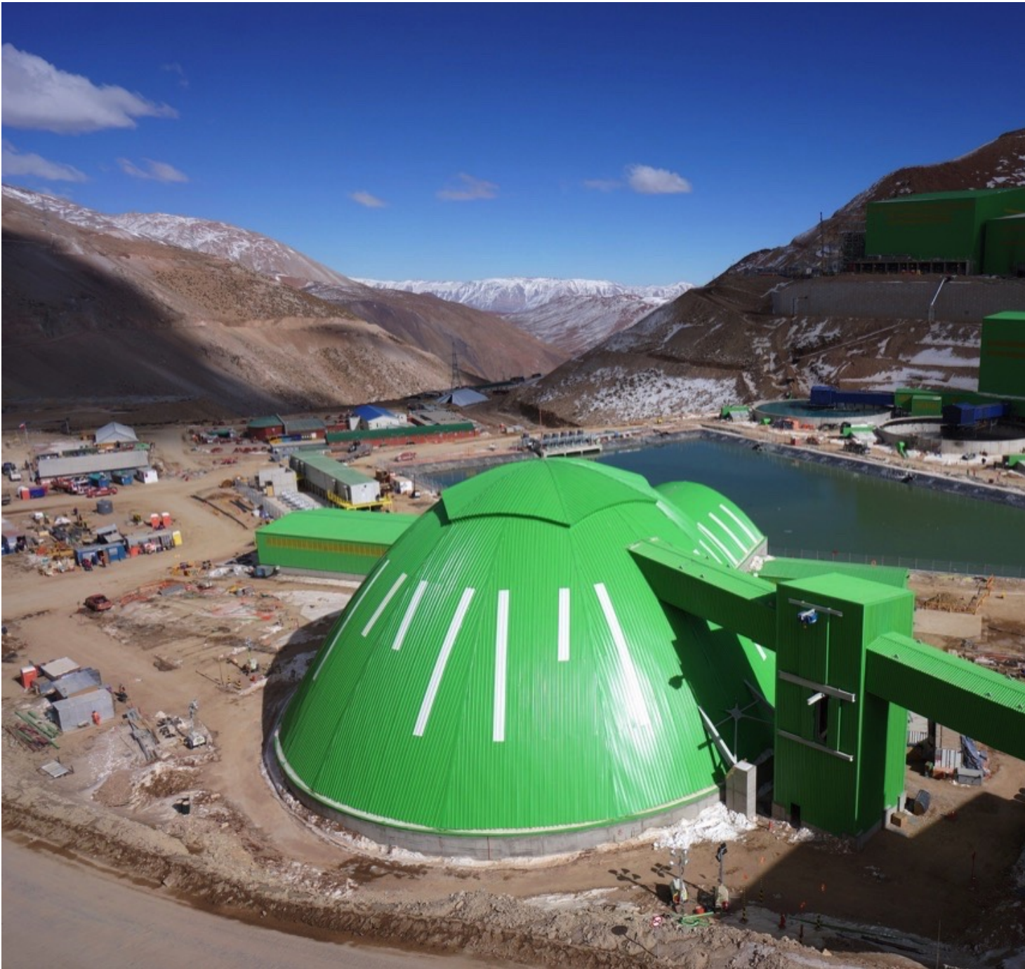
High winds, punishing snow loads, and torturous slopes at 4000 m above sea level in the Chilean Andes.
