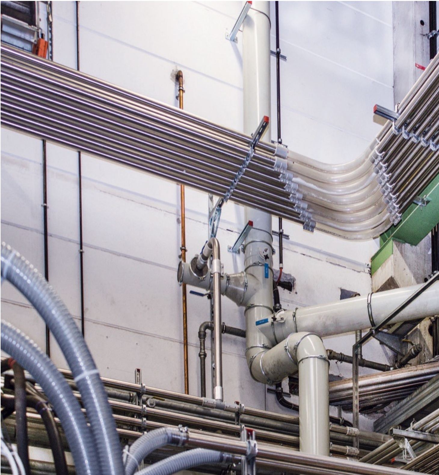
Shut-off valves were installed at strategically important points in order
