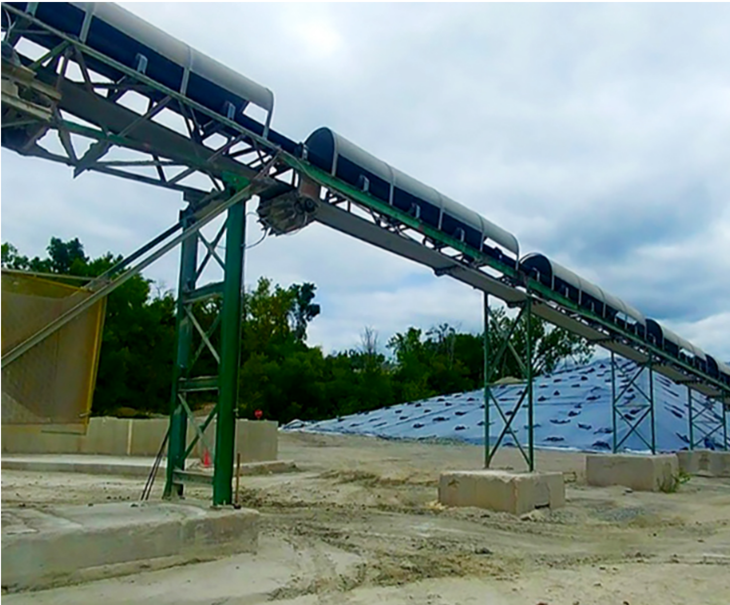
The 107-1 conveyor rises 20 feet (6 m) at its mid-section.
