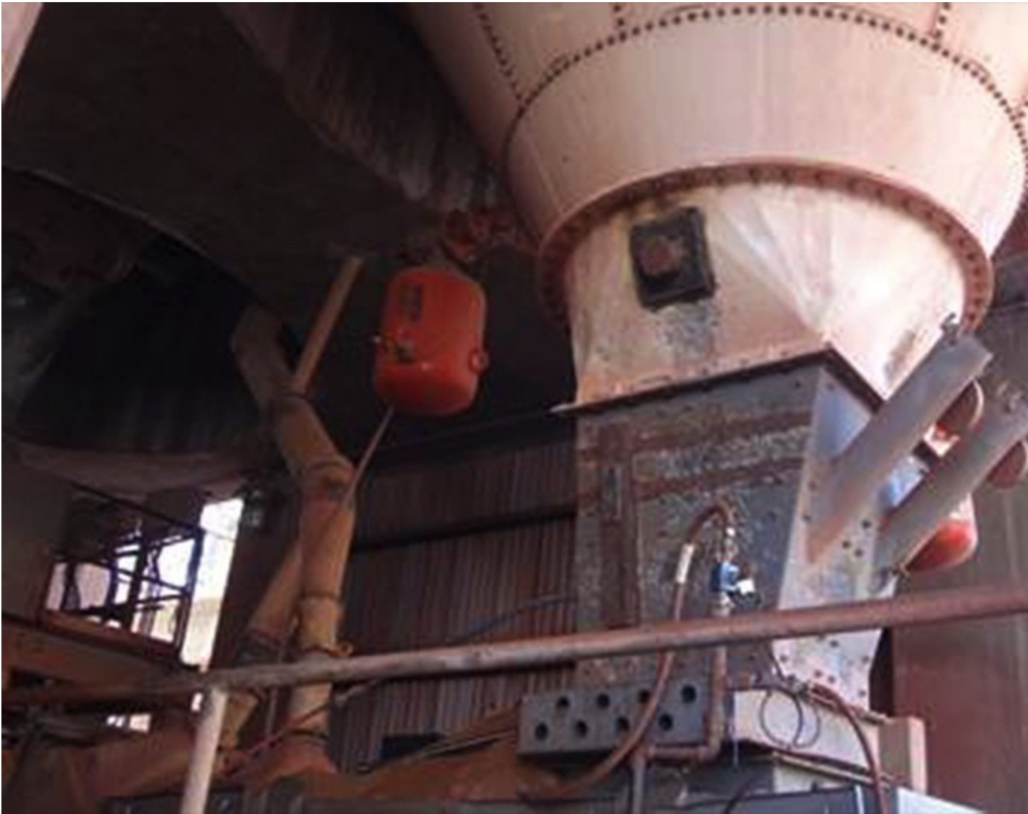
Martin XHV air cannons at Drake cement in their original perpendicular firing configuration (Pictures: © Martin Engineering)
