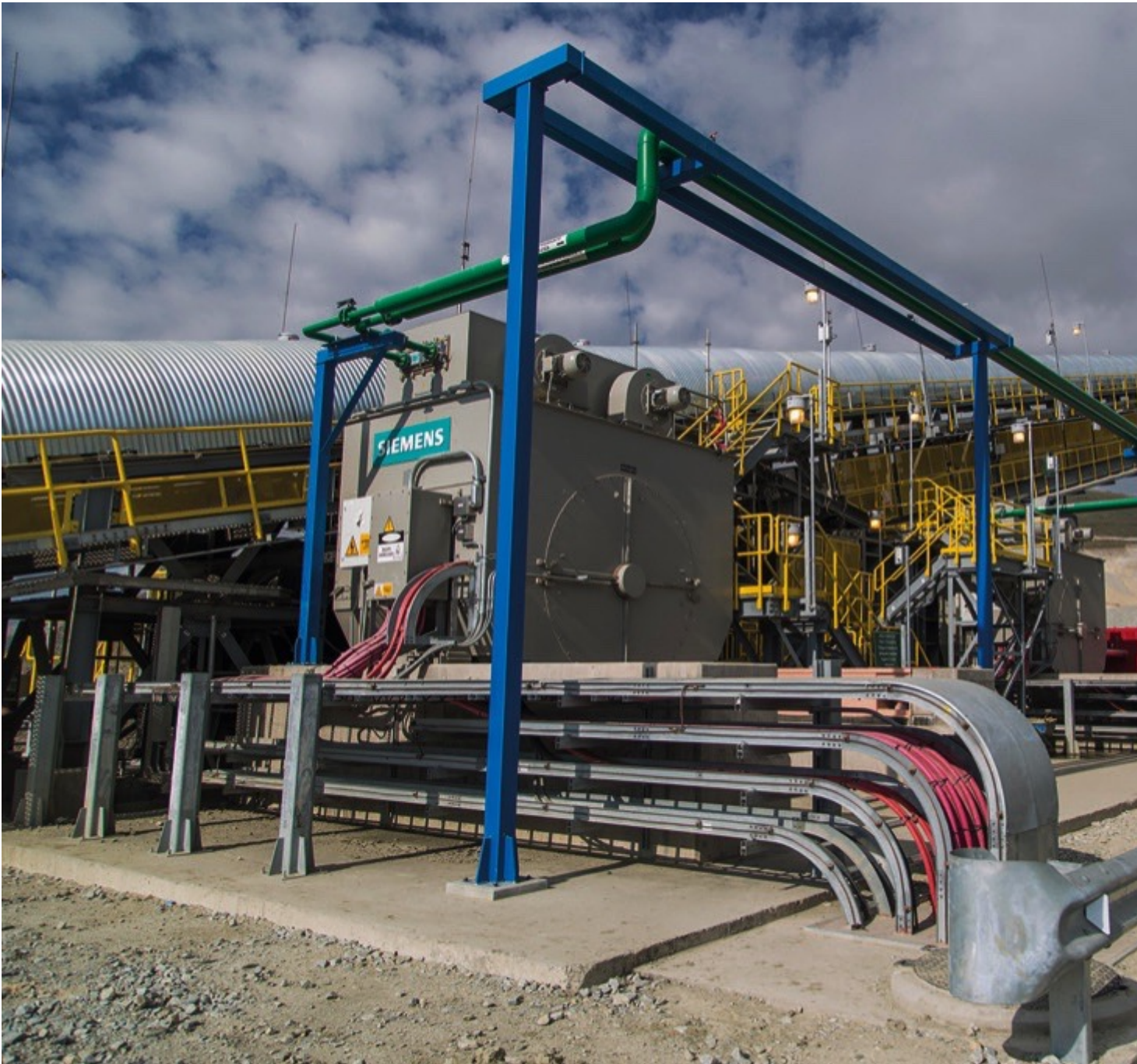
Fig. 13: Direct drive for a belt conveyor, 2 x 4.4 megawatts.
