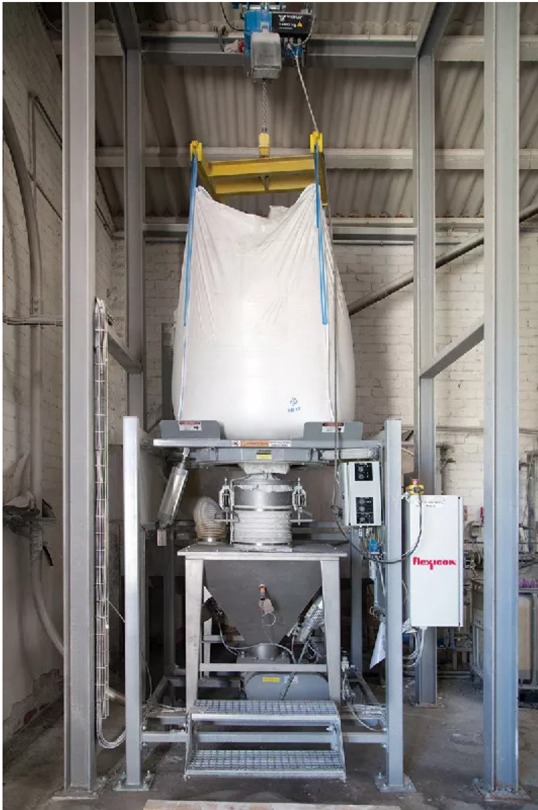
The powder flows dust-free into the hopper and into the following 38 m long pneumatic transfer line.
