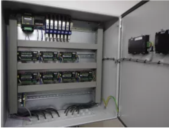
Fig. 3: View into the electrical cabinet: control unit ModWeigh FBW
