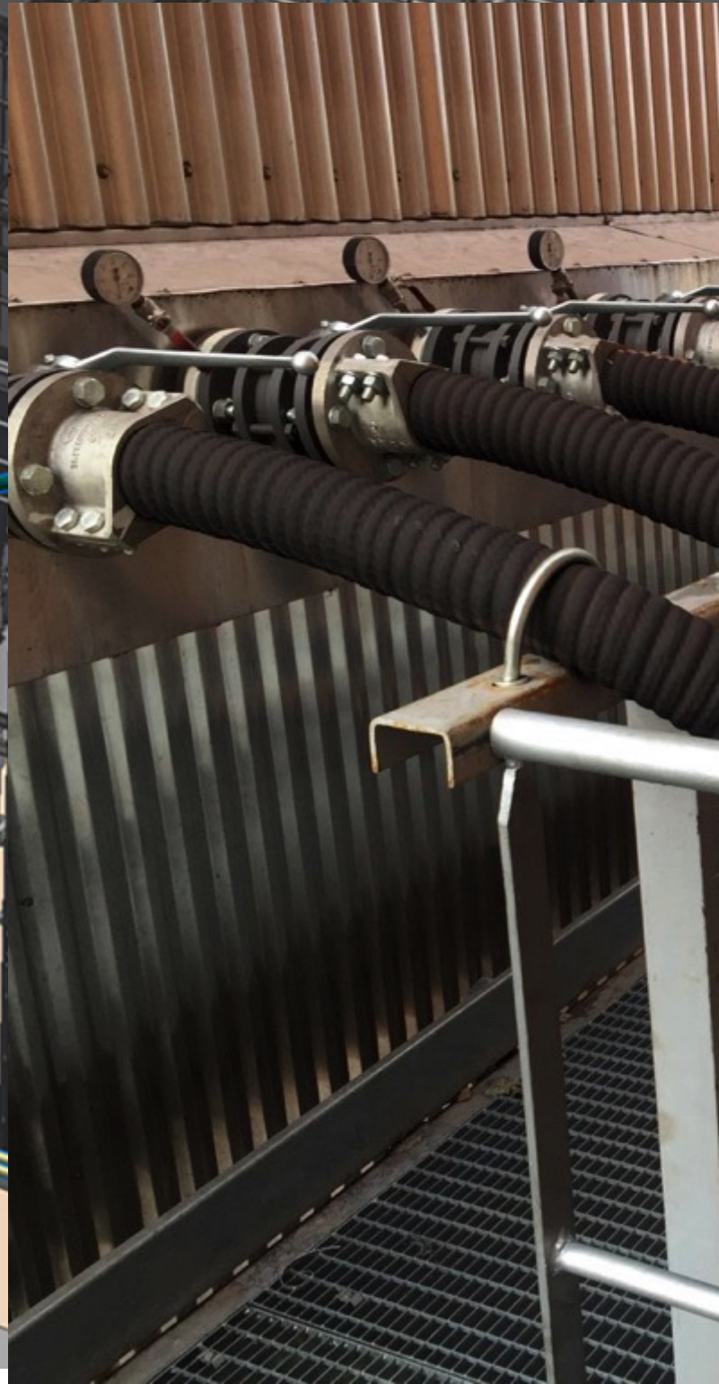
Fig. 16: Sixteen Injectors supplied by two 8-fold pneumatic conveying lines.
