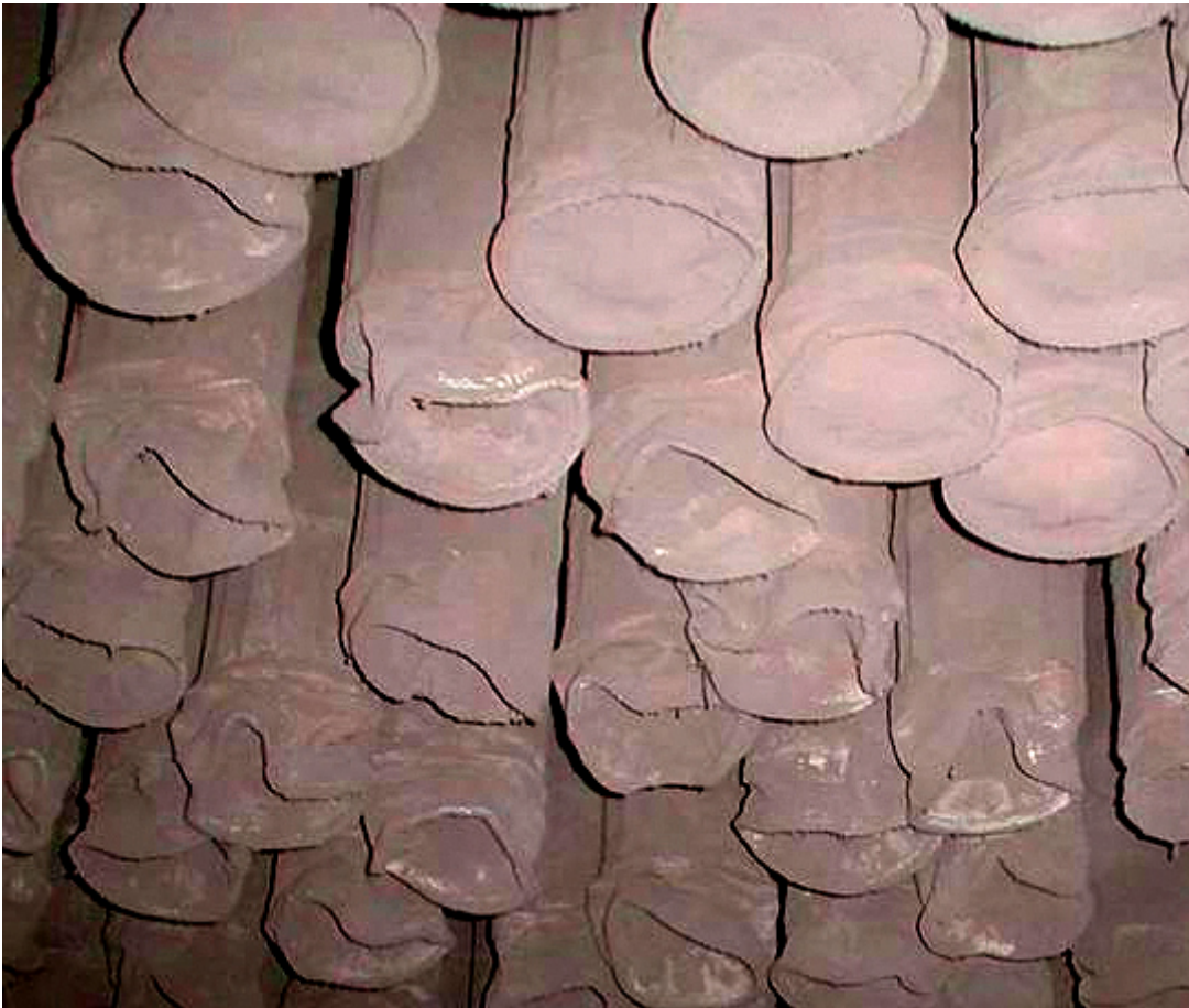
Fig. 10: Photograph from “Why bags fail”: View into a bag house. (Picture: ©Heimbach Filtration GmbH)
