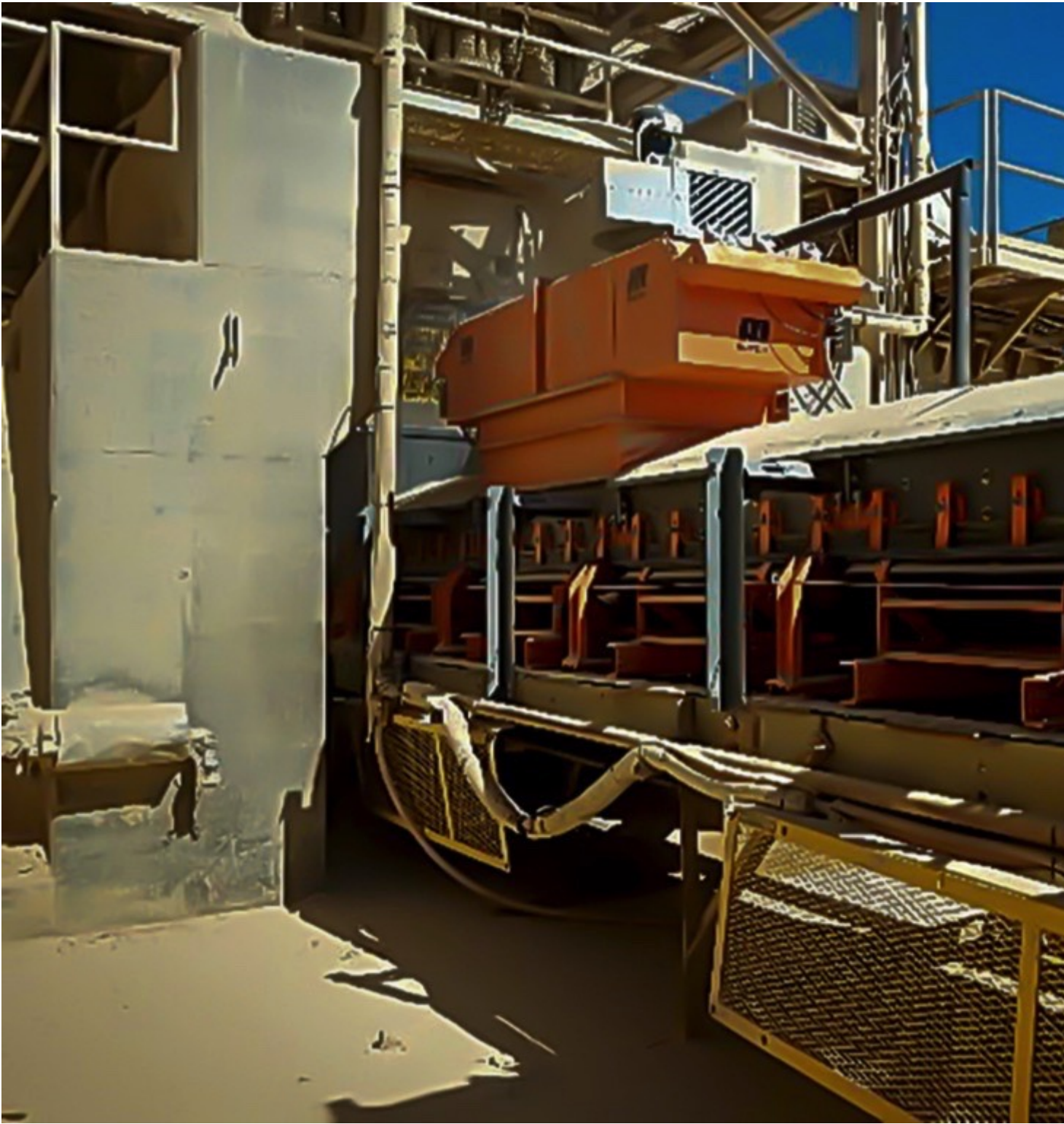
Fig. 7: The integrated air cleaner is an independent unit positioned directly at a dust generation point. (Picture: © Martin Engineering)
