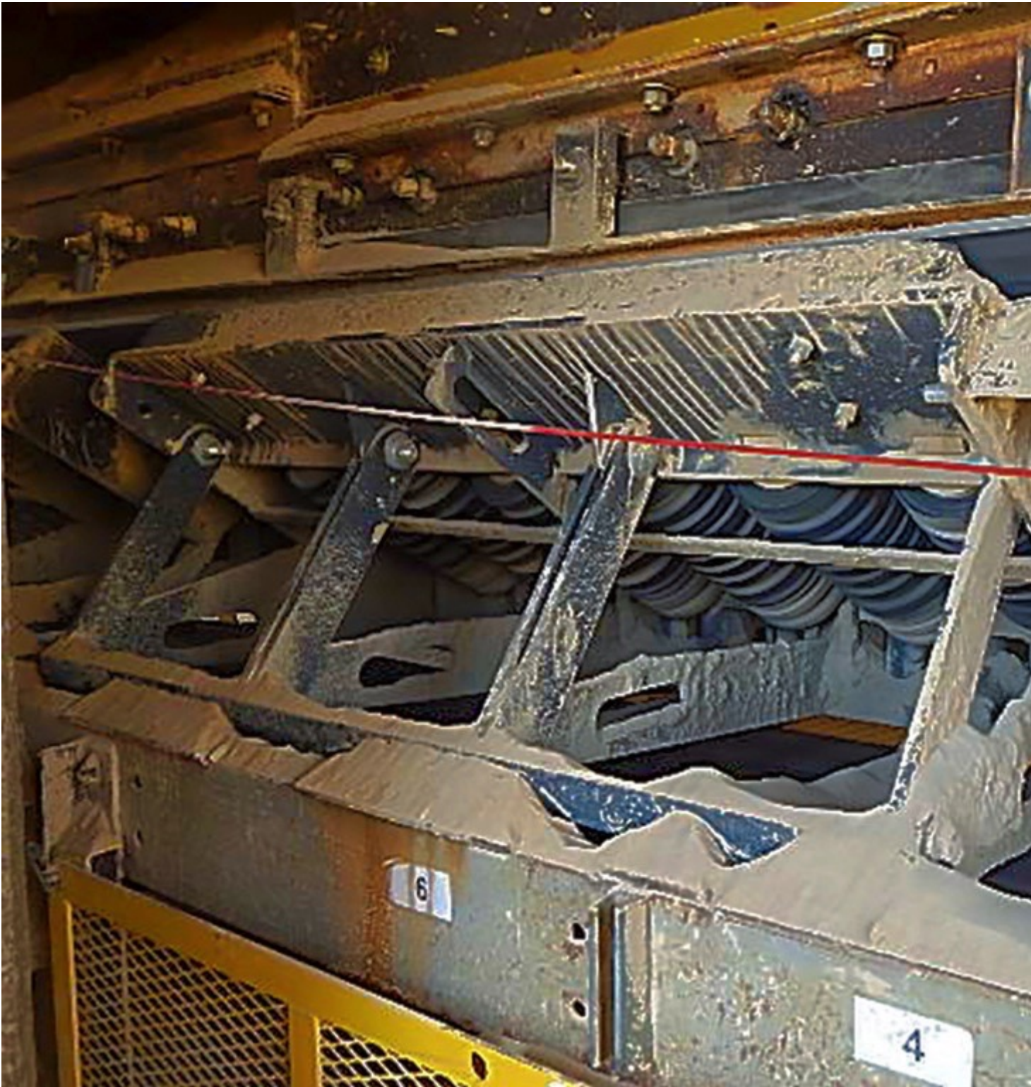
Fig. 2: Dust and spillage created a maintenance burden and potential safety hazard (Picture: © Martin Engineering)
