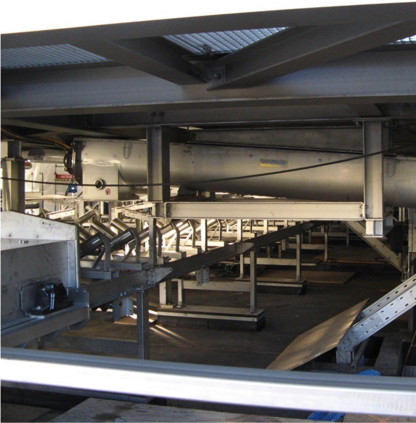
Van Beek Screw conveyors after installation at the Geleen Ammonium Sulfate plant (Picture: © Van Beek B.V.)
