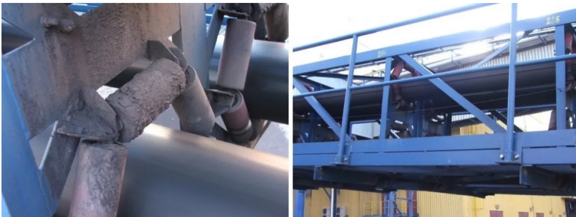
Fig. 2. Example of situation when the conveyor belt does not have a contact with all idler rolls in the hexagonal idler housing.
