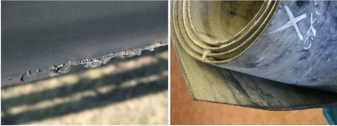
Fig. 1. Example of damage on edge of the pipe conveyor belt. (Pictures: © Technical University of Košice)
