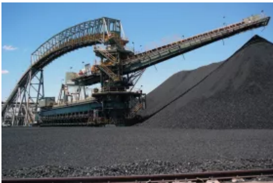
Circular storage and blending bed by Schade for BHP Blackwater mine Australia.
