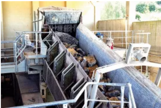
Apron plate feeder for raw material intake to crushing plant.
