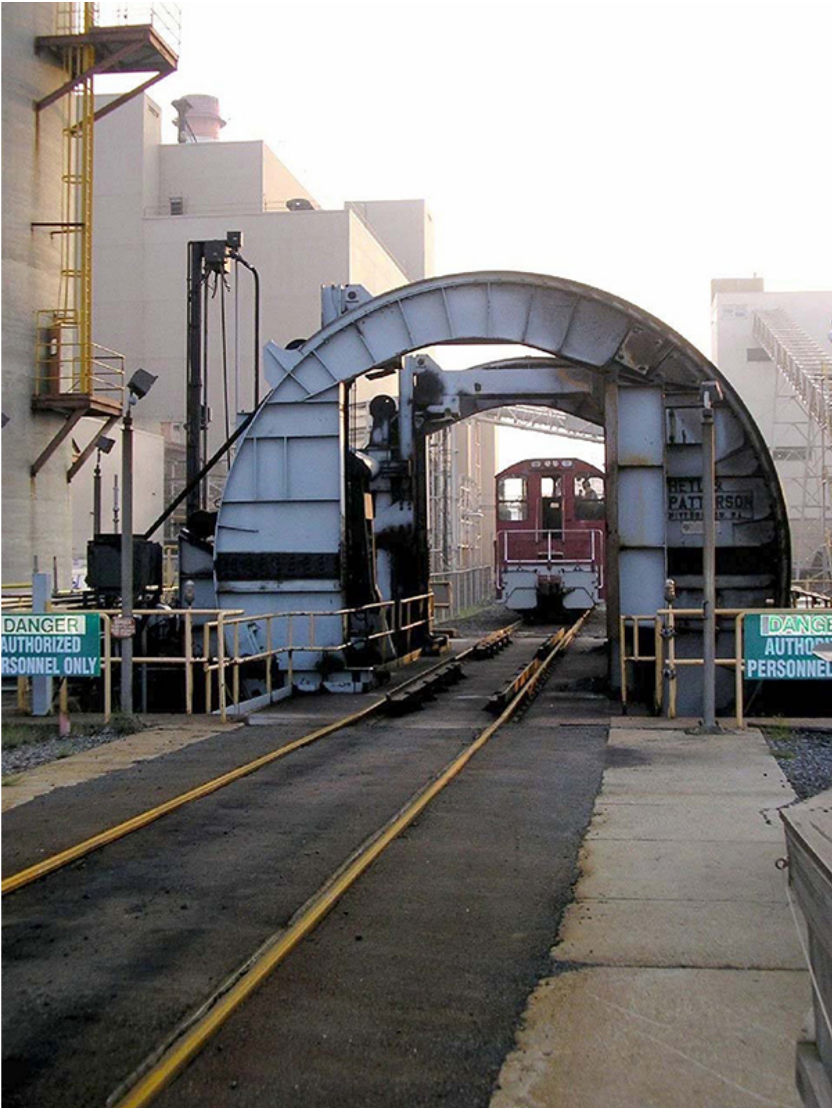
A train is approaching the railcar dumper at an iron ore smelter. (Pictures: © Heyl & Patterson)
