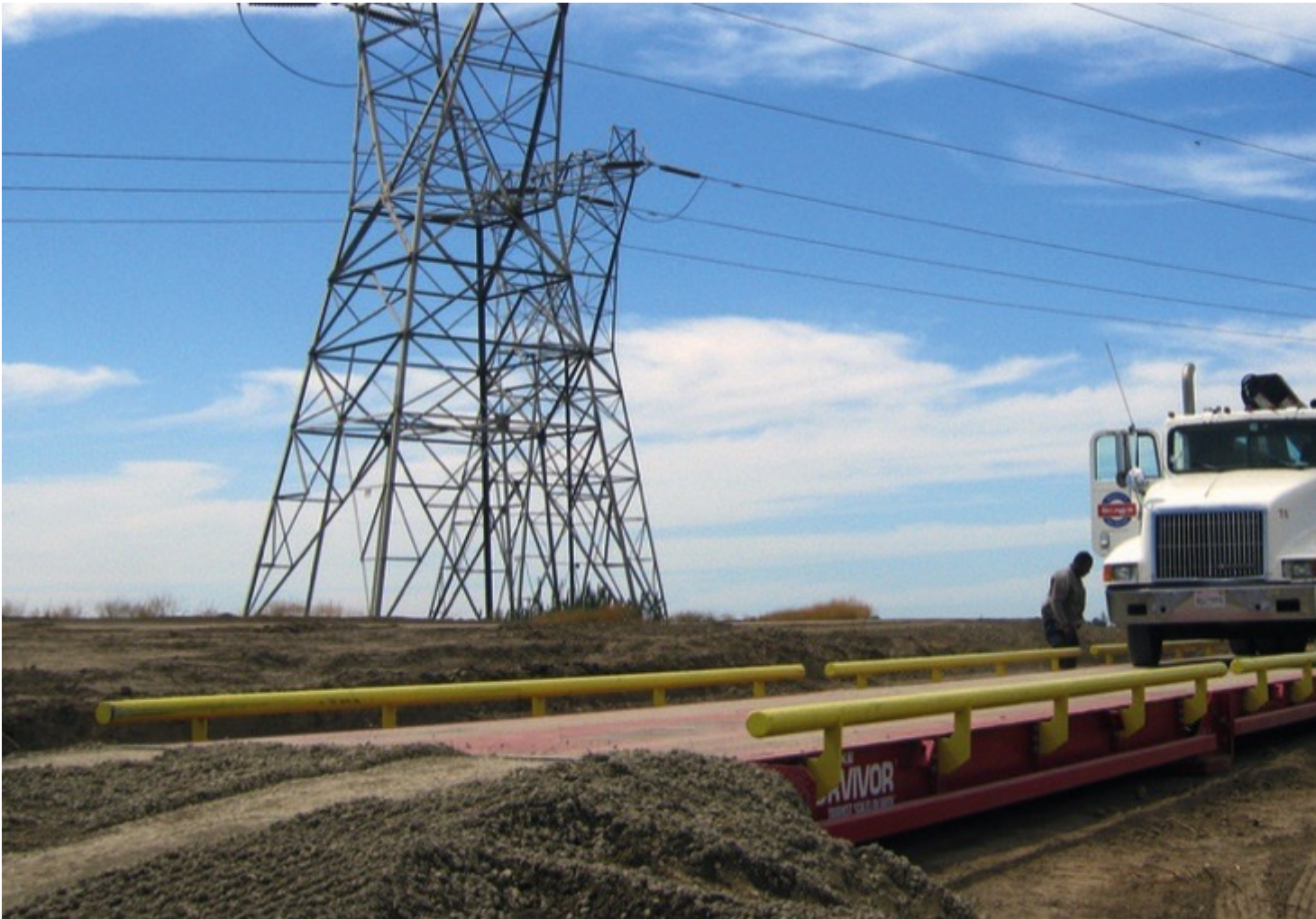
Above-ground installation of a belt scale. (Pictures: © Quality Scales Unlimited)
