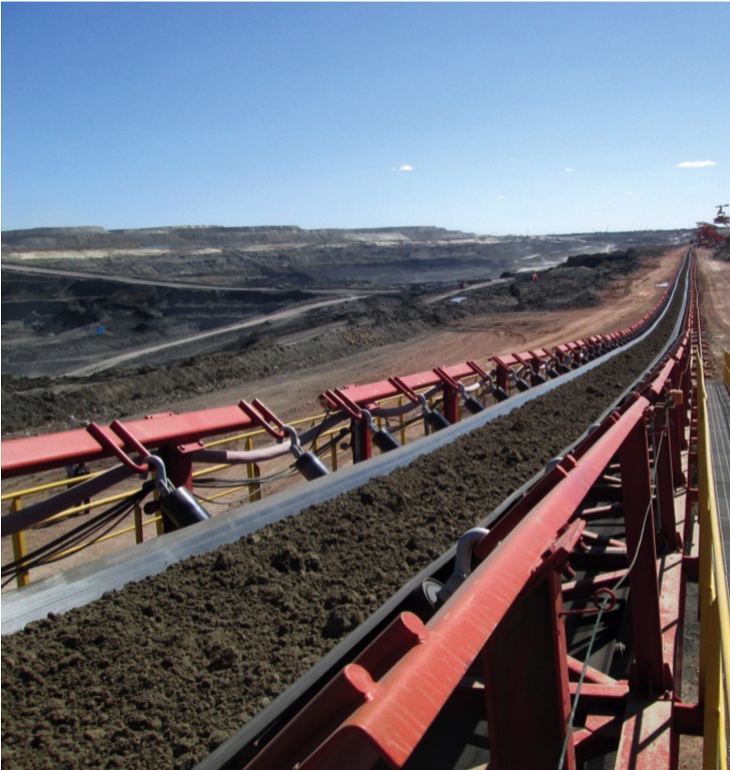
7900 m 3 /h Tenova Takraf conveyor system at Zhahanaoer open pit mine in China.
