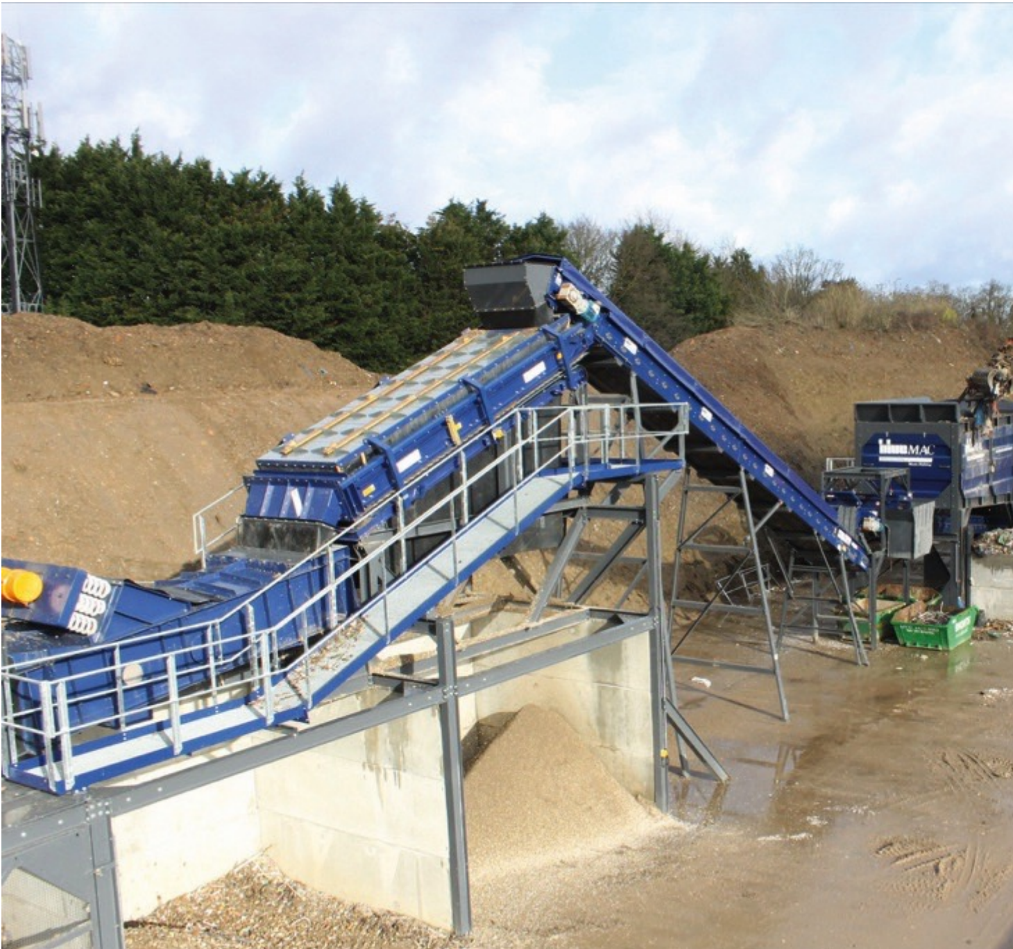
Bluemac erected a bespoke MRF for Shorts Group in Ascot. (Pictures: ©Bluemac Manufacturing)
