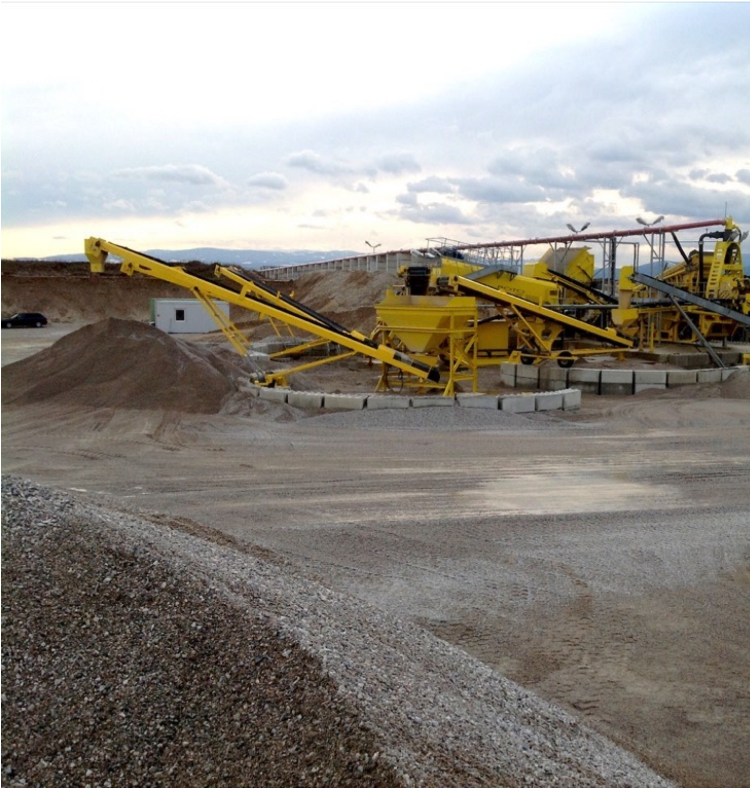
The new gravel washing plant of Pehofer in Wiener Neu-stadt, Austria (Pictures: ©CDE Global, Pehofer)
