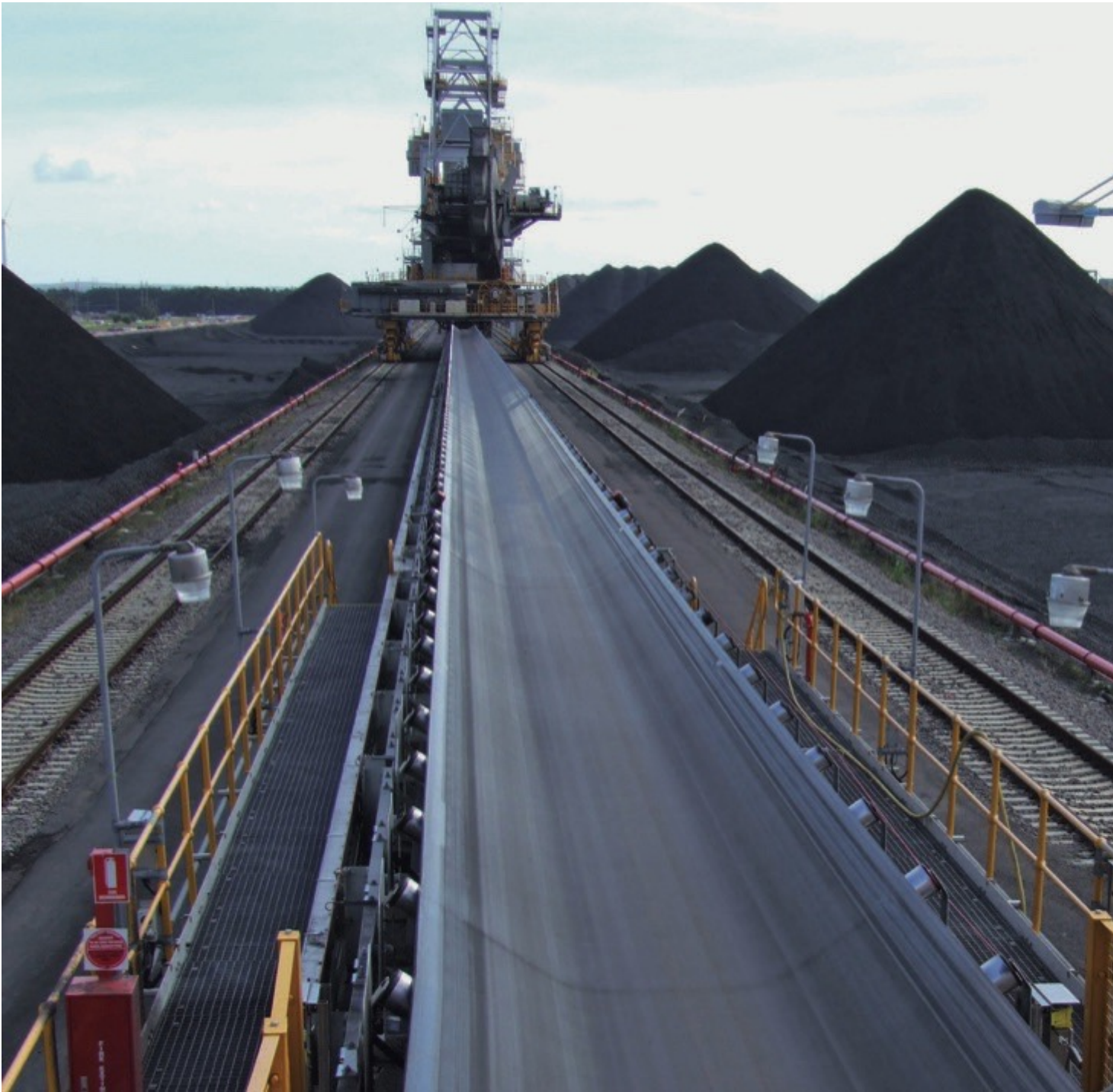
Fig. 1: At NCIG's coal terminal the principal conveyor belts are 2.5 metres wide, working with high tonnages, where current capacities can reach up to 33 million tonnes a year.
