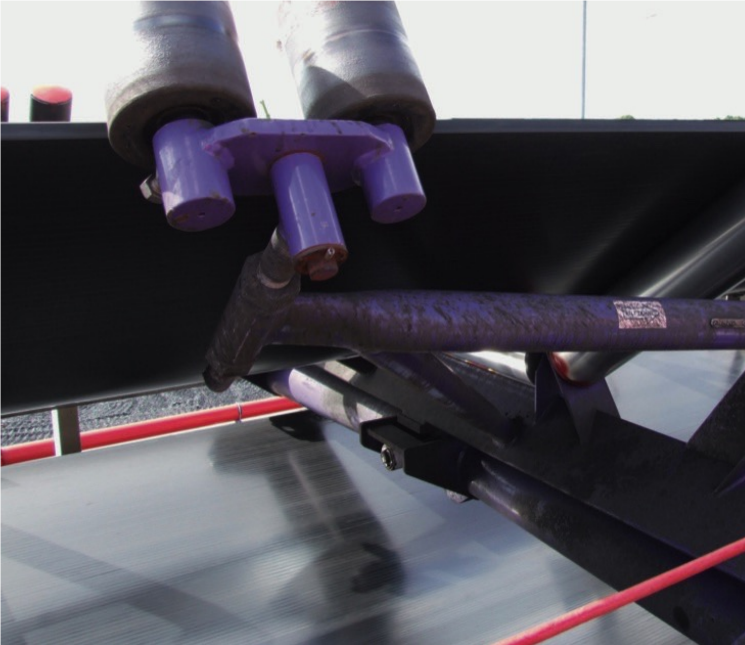
Fig. 2: Heavy duty PT Max belt trainers were used to resolve the recurring tracking problems at the terminal.
