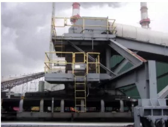
Fig. 2: The old chute would build up and plug with coal fines that stuck together when in wet coal or freezing conditions.
