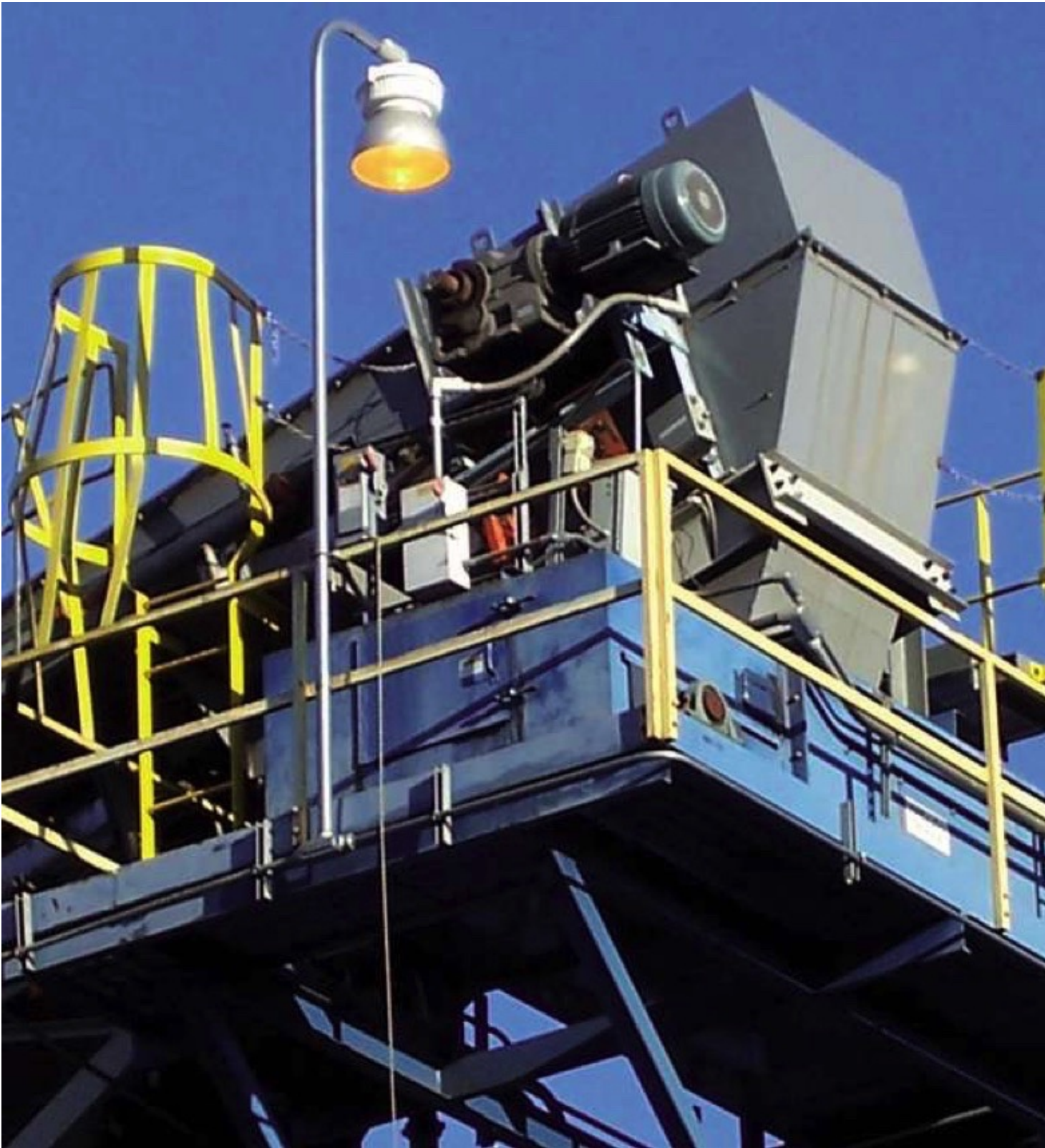
Fig. 1: This section of existing air-supported conveyor leads to a field-fabricated head chute with brush belt cleaners to mitigate dust and plugging. (Pictures: © Martin Engineering)
