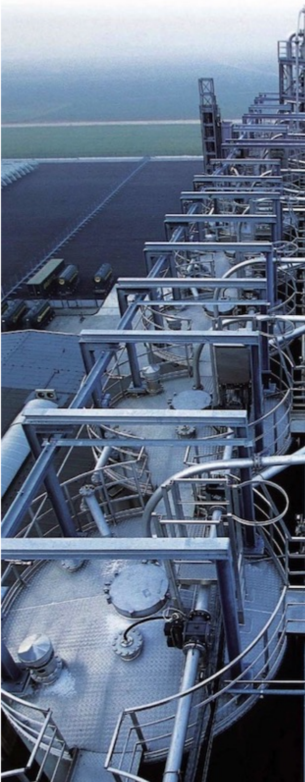
Fig. 3: Each plant is subject to specific requirements and is individually designed and built.
