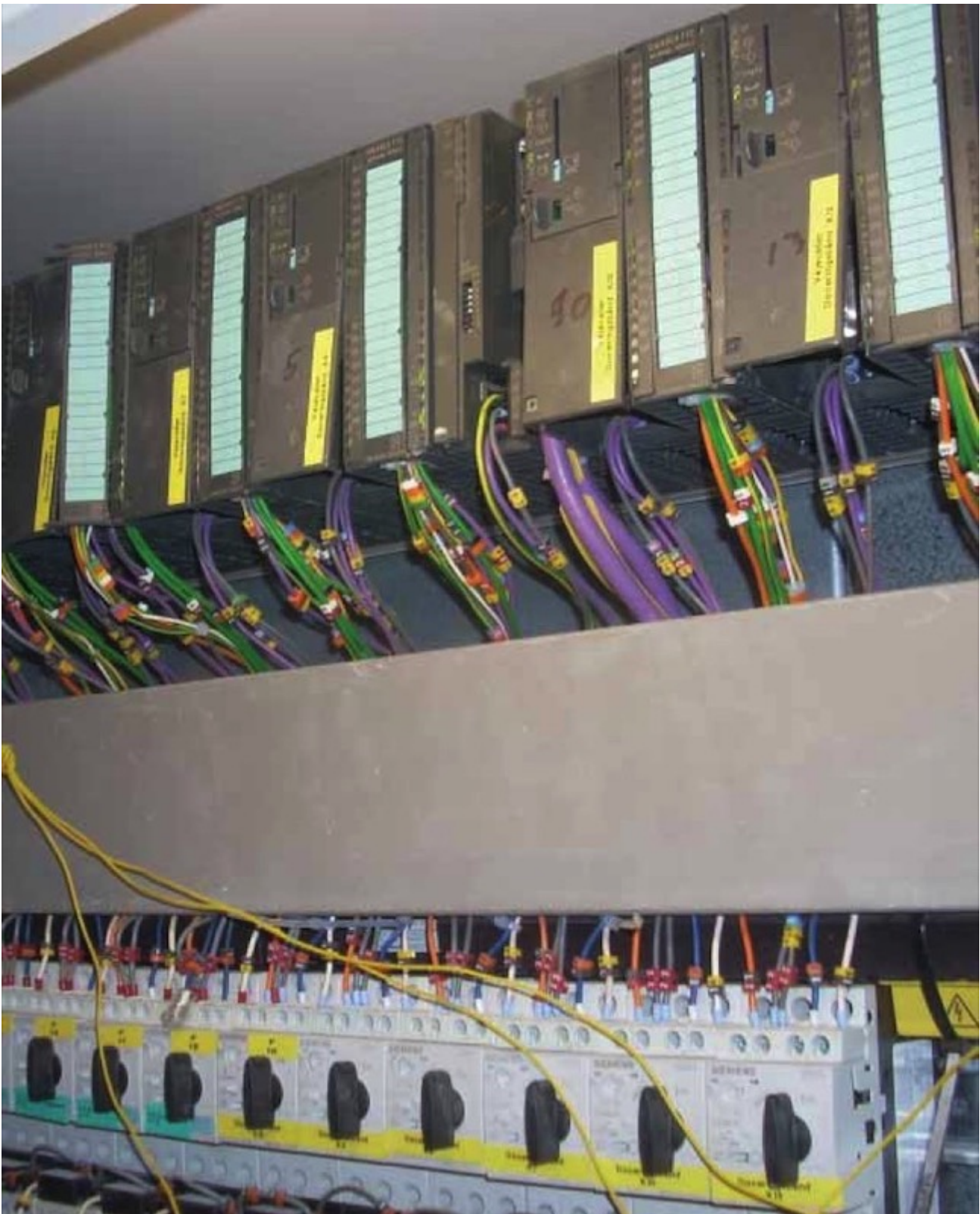
Fig. 2: Siwarex FTC weighing modules during commissioning they provide fast, continuous monitoring and control delivered directly to Nopa's control room.
