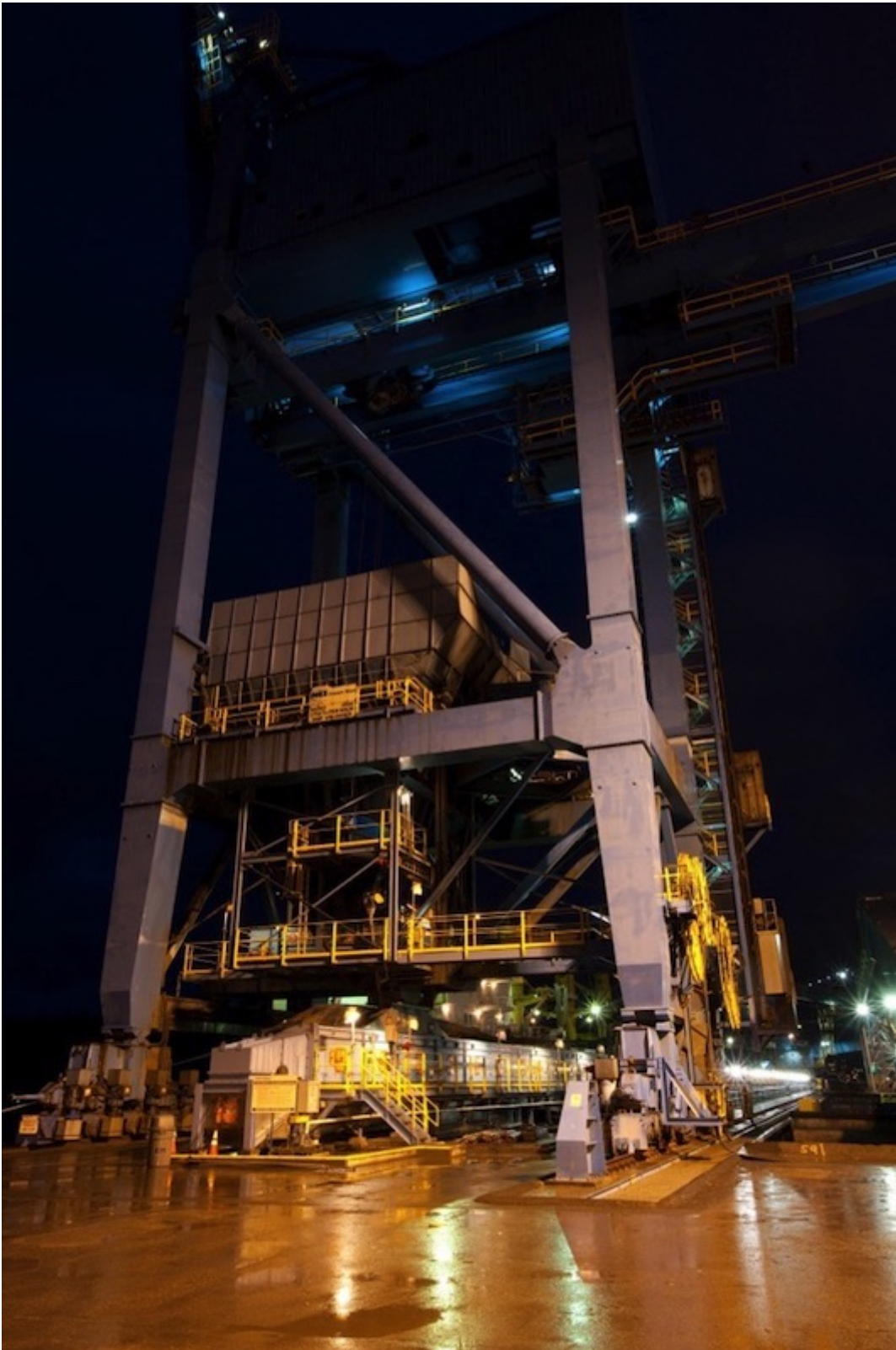
Fig. 1: A load-out hopper and four belt conveyors with capacity for 1500 tonnes per hour of mineral ore concentrate have been installed at the Kinder Morgan North Vancouver facility.
