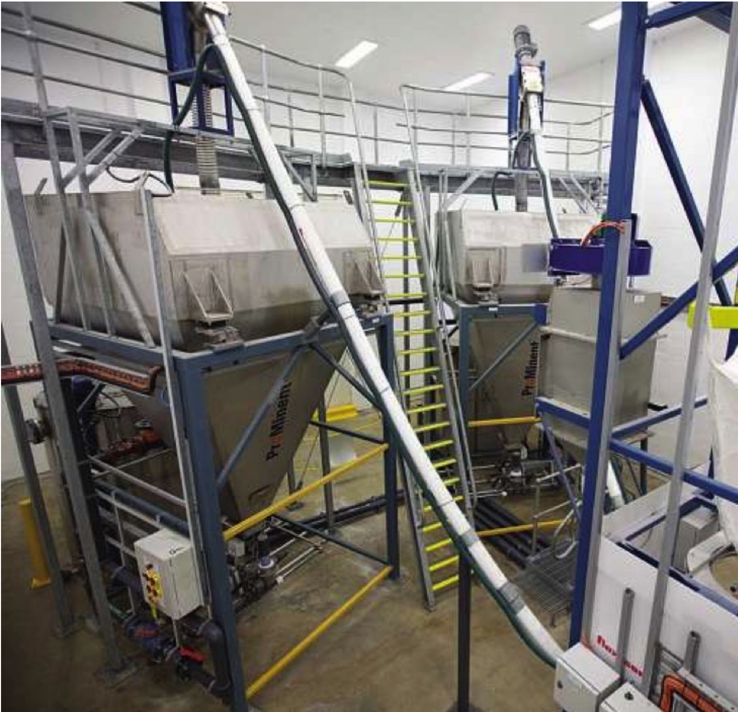
Fig. 1: Recently, Prominent Fluid Controls has supplied equipment for large water-fluoridation plants; the major pieces of equipment are a bulk bag discharger, a dust containment system, and a flexible screw conveyor. (Pictures: ©Flexicon (Europe) Ltd.)
