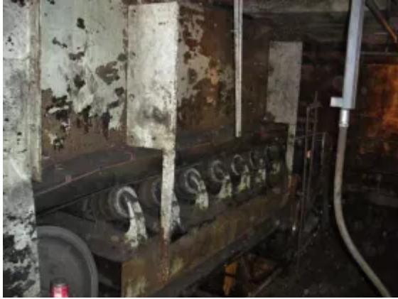
Fig. 1: MCGS took a proactive approach to upgrading conveyor feed systems, conducting a plant-wide assessment.
