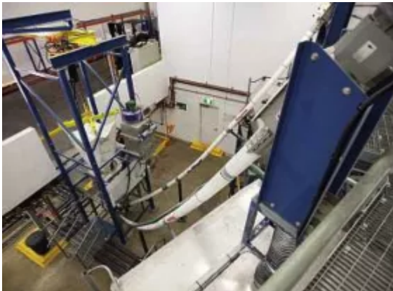
Fig. 3: Powder remains enclosed from the time it is received until it enters the mixing tanks.
