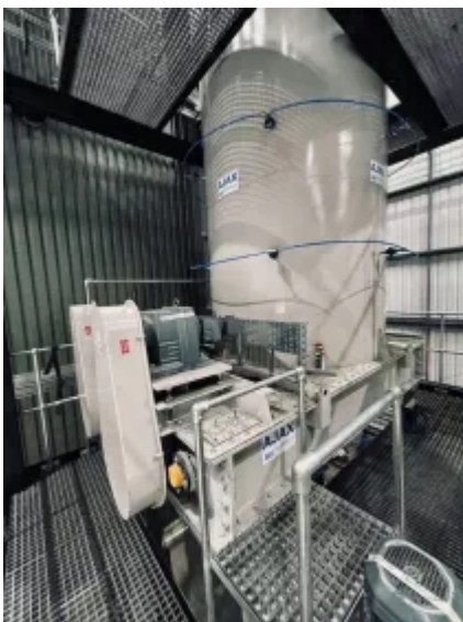
Ajax's carbon fibre handling system installed at Mersen.
