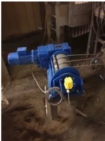
The bespoke electric winch used for the safe and smooth lifting and lowering of a large telescopic export chute.
