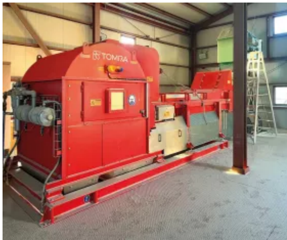
OMRA COM Tertiary XRT installation
