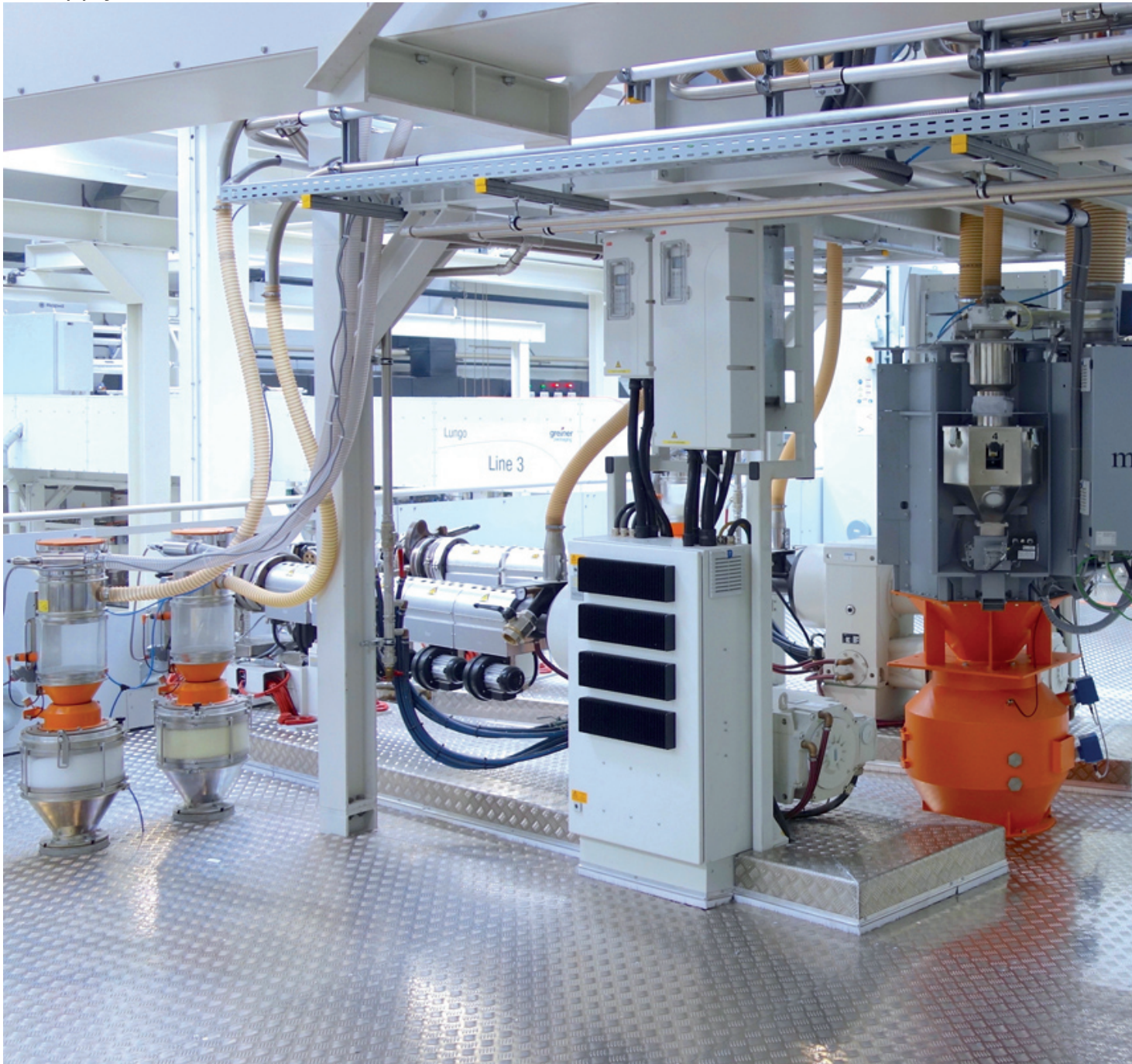
Fig. 5: Central mixing station to supply the “regrind extruder”. In this, four material components come together (regrind from the silo or from the BigBag, stabiliser for the adhesion promoter and new PP material) which are added from the gravimetric dosing
