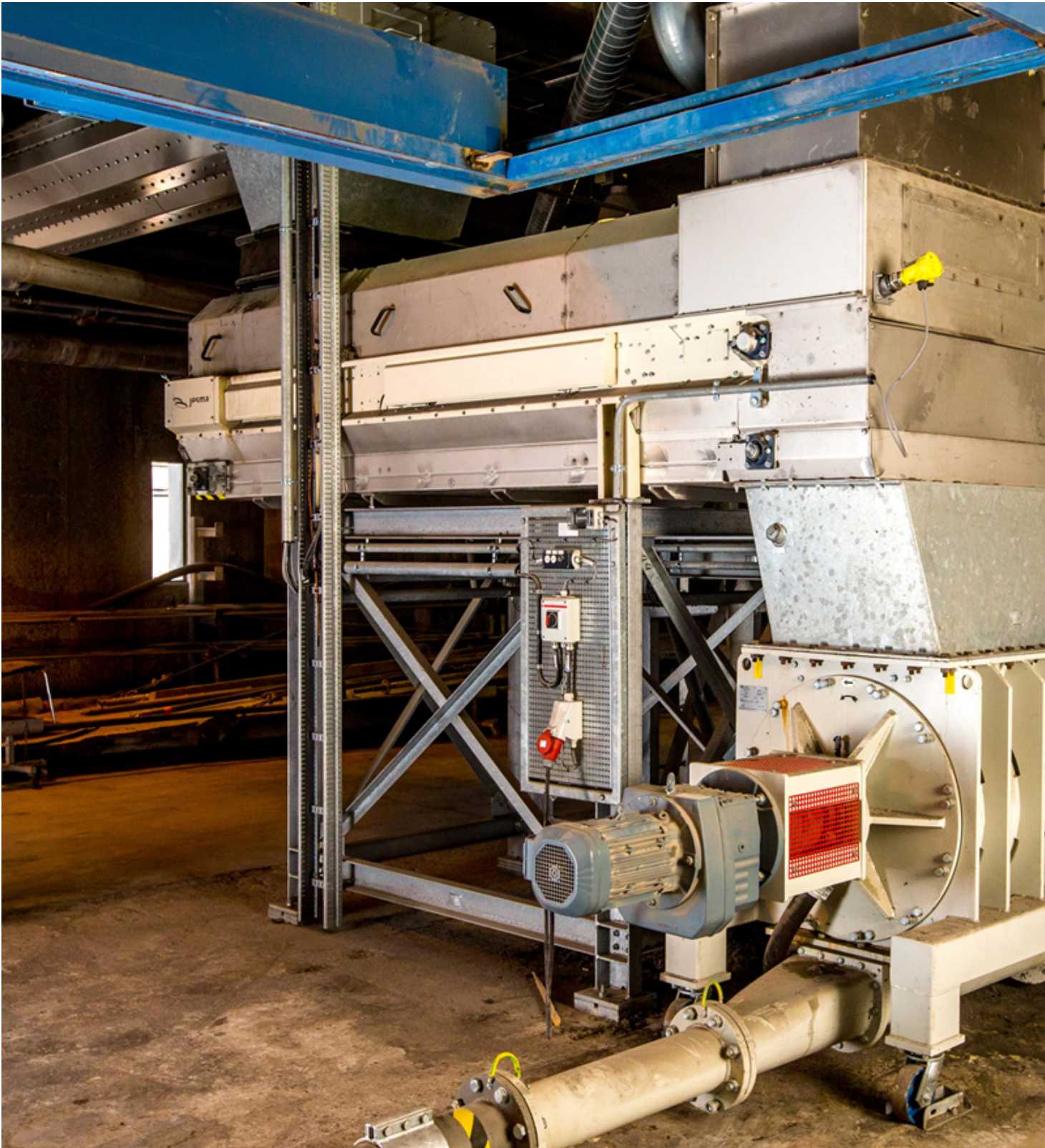
Fig. 6: The weigh belt feeder with the rotary vane feeder including a blower conveys the material to the main burner through the pipes in a pneumatic way. (Picture credits: BEUMER Group GmbH & Co. KG)
