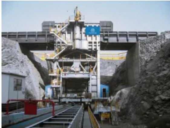
Direct feed semi-mobile crushing plant at a Chinese iron ore mine.
