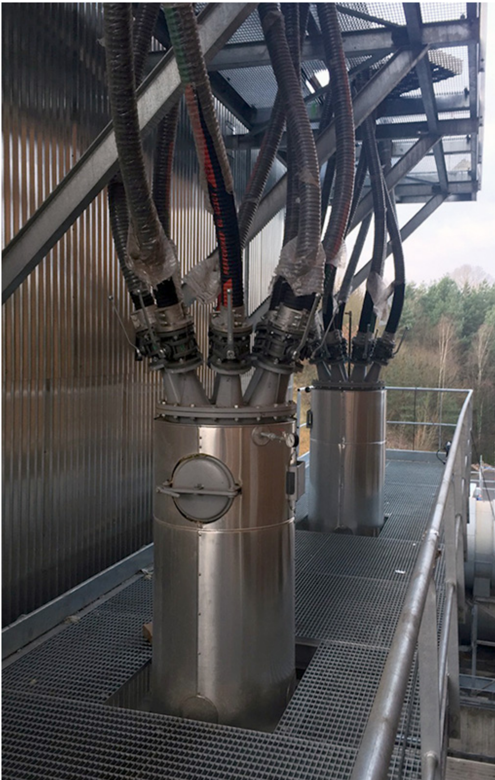
Fig. 17: Two splitters, supplying eight pneumatic injection lines each.
