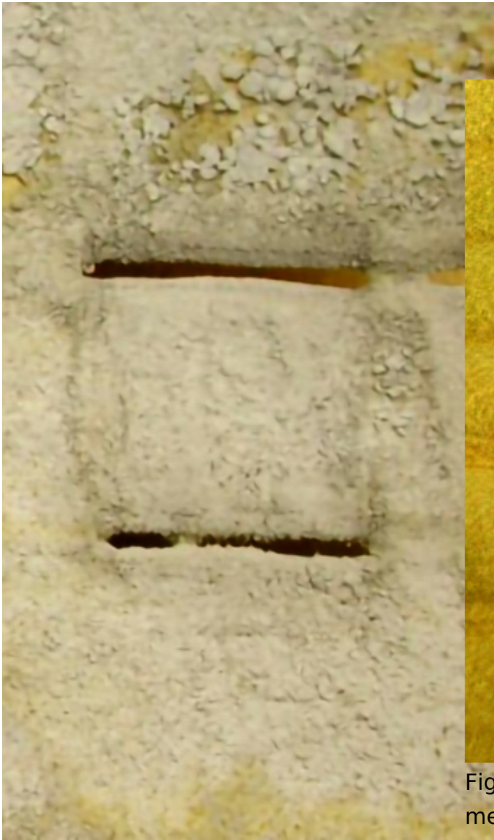
Fig. 8: Hole along cage wire uncleaned (left) and cleaned (right).
