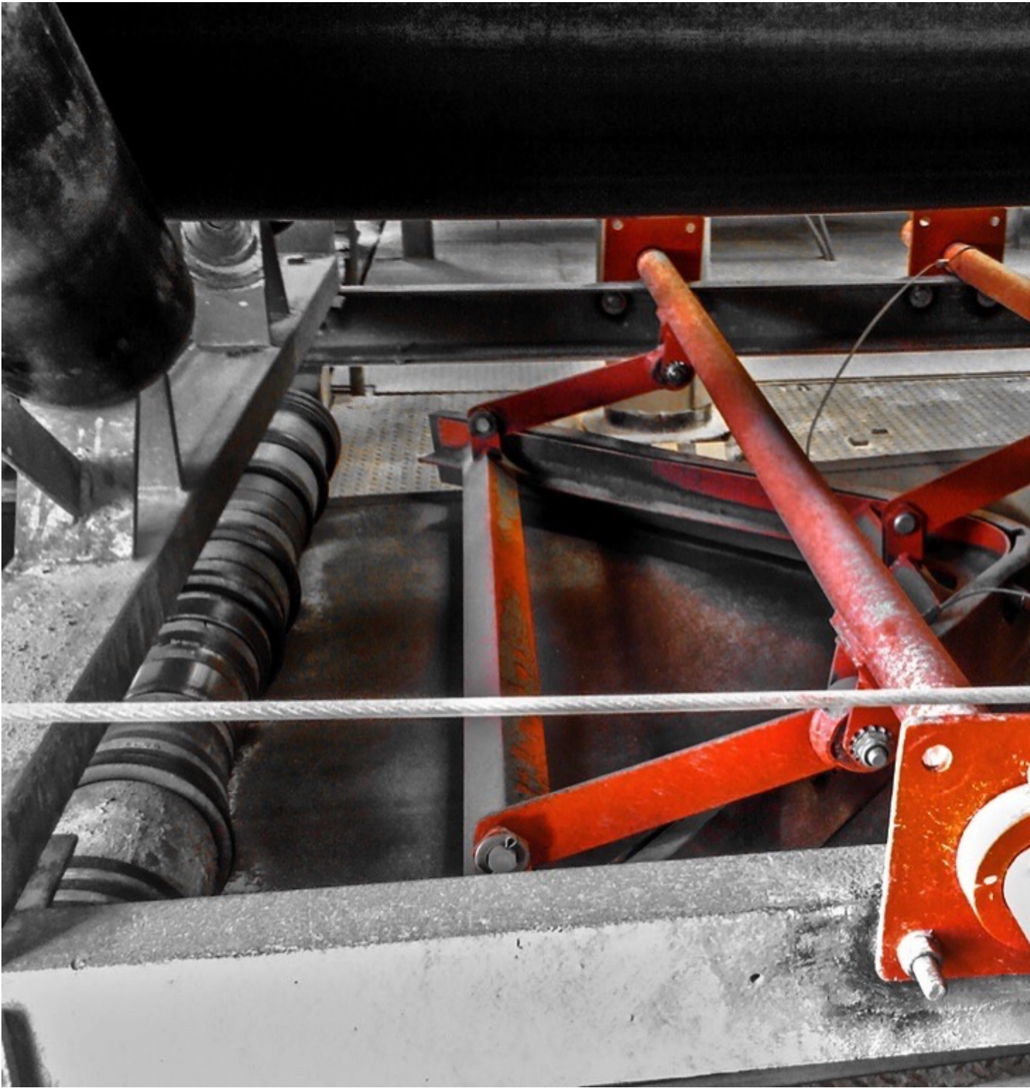
Fig. 6: The V-Plow features spring-loaded suspension to rise and fall with fluctuations in belt tension and travel. (Picture: © Martin Engineering)
