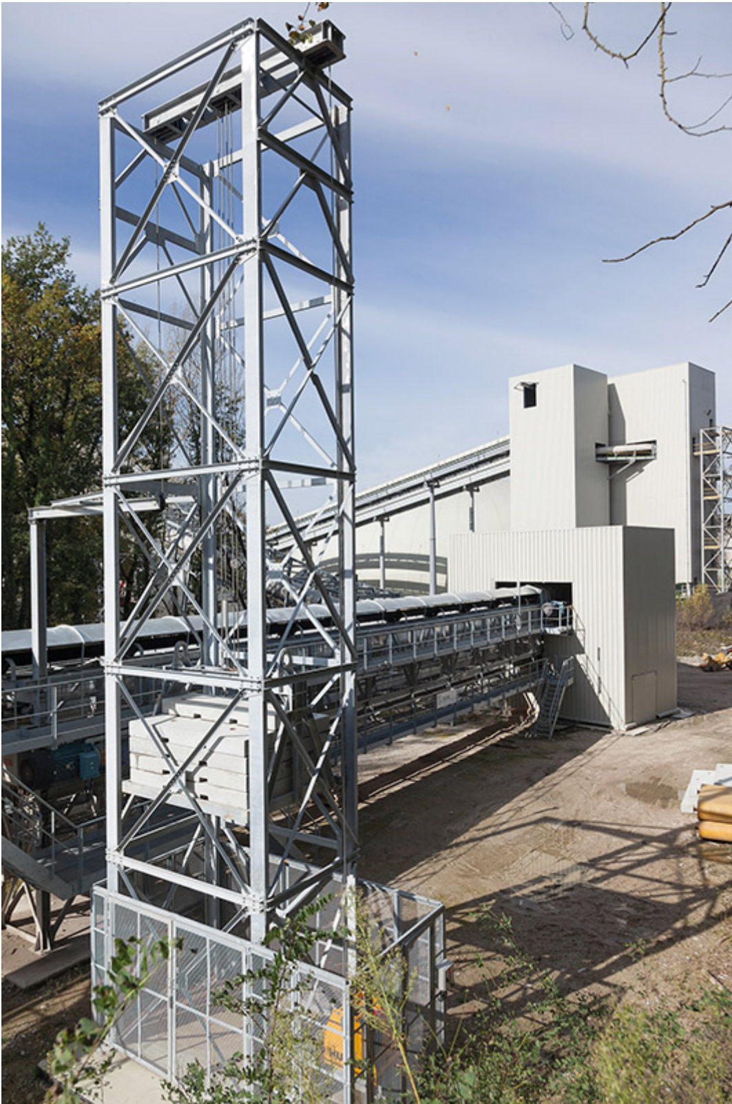
Headstation of the Vicat conveyor. The steel tower contains the belt tensioning system. (Pictures: © Contitech, Techmi)
