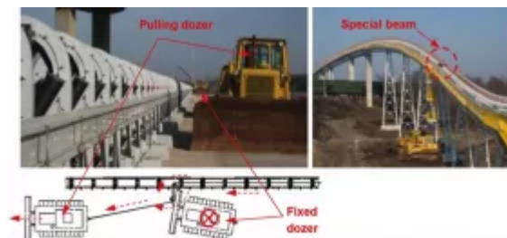
Fig. 13: Belt pulling-in process on the ground (left) and at a high elevation of the system (right).
