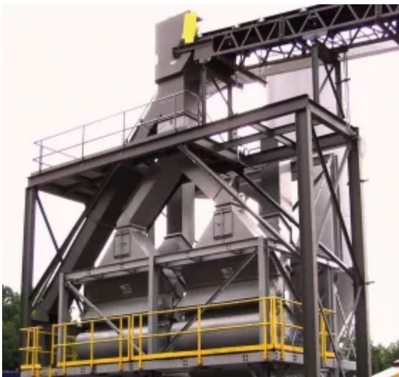
Fig. 10: Metso's Dual AC22.5GI static air-classifier units at Luck Stone's Goose Creek plant, operating at maximum throughput of up to 100 tph. (Picture: © Metso Minerals)
