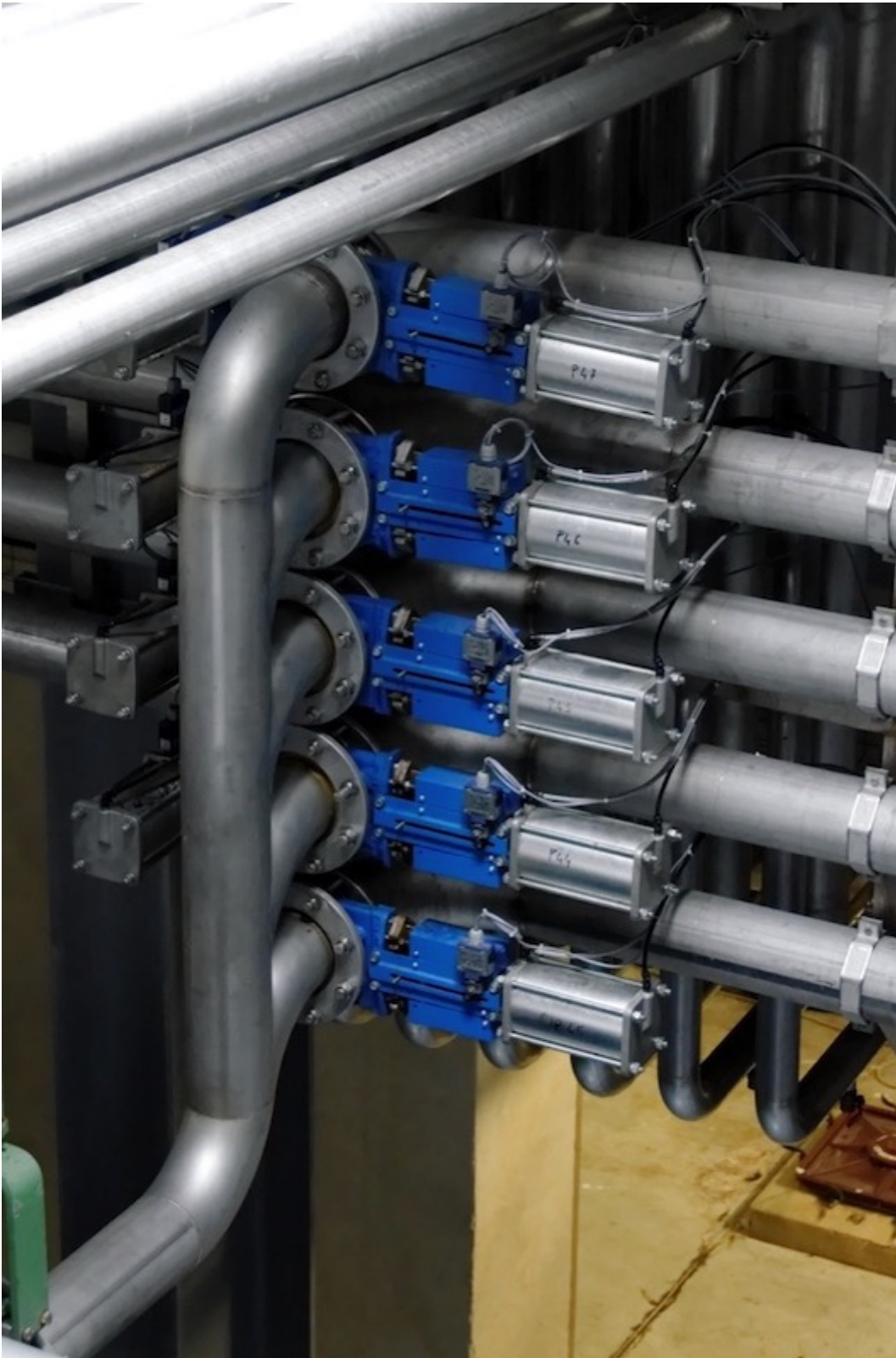
Fig. 1: Pneumatic conveying systems have a number of advantages; one of the disadvantages, however, is the wear in pipe bends. (Picture: yelkrokoyade, CC By-sa 2.5)
