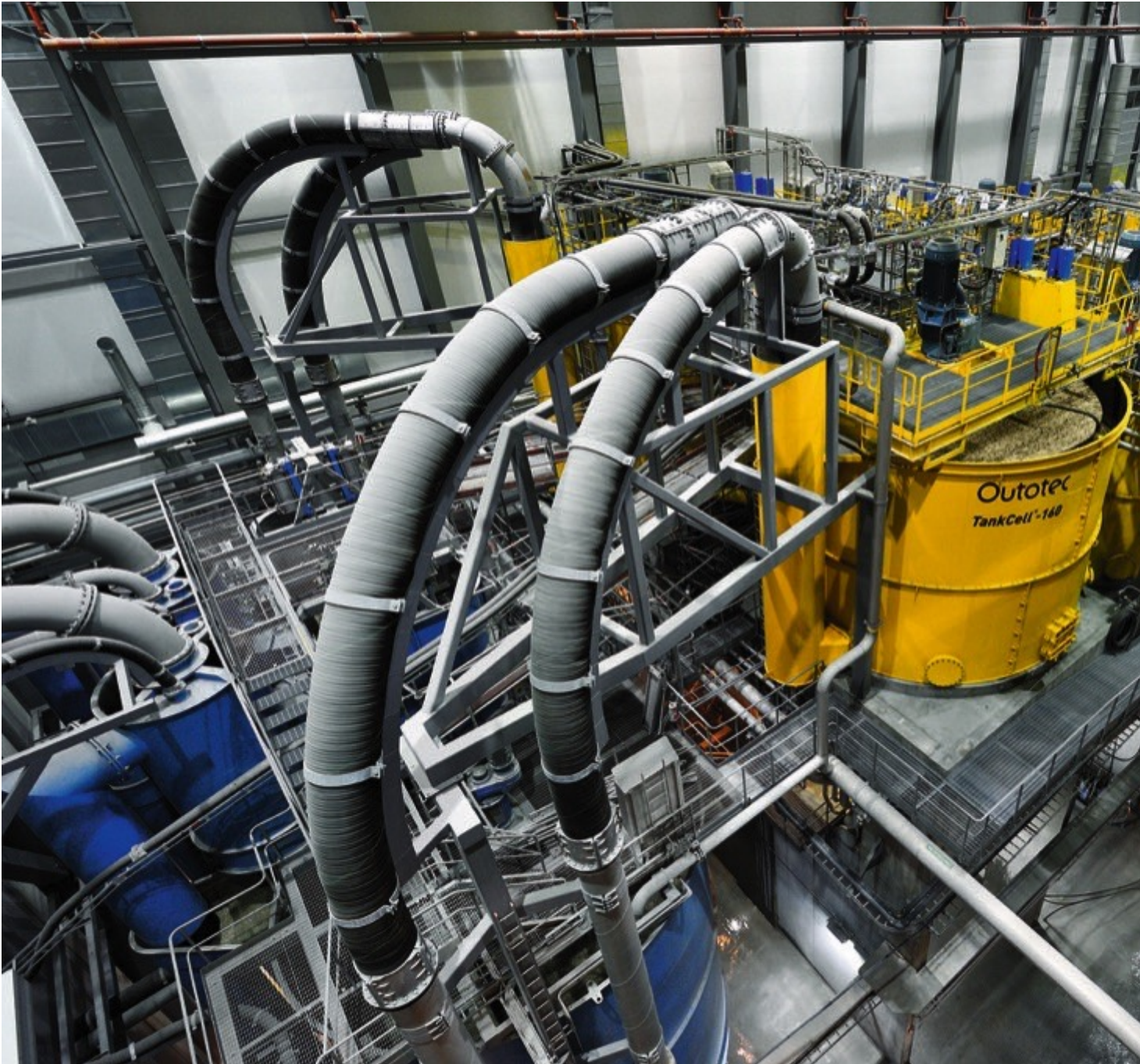
Fig. 1: With the new asset management system, Boliden handles the information of about 4500 instruments at its Aitik mine in Sweden. (Pictures: Endress+Hauser)
