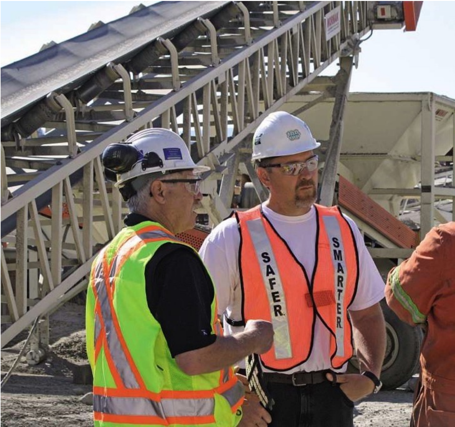
Fig. 1: Owners and operators that are around the conveyors every day may not notice the slight changes in the system, while a fresh set of eyes can identify issues. (Pictures: ©Flexco)
