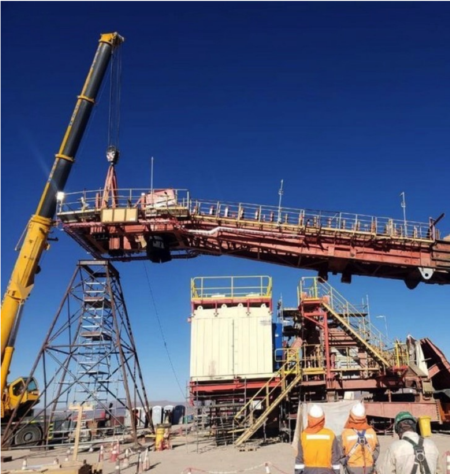
Installation of the boom into the superstructure of the TAKRAF BWR 7100 at the mine in Chile. (Picture: ©TAKRAF)
