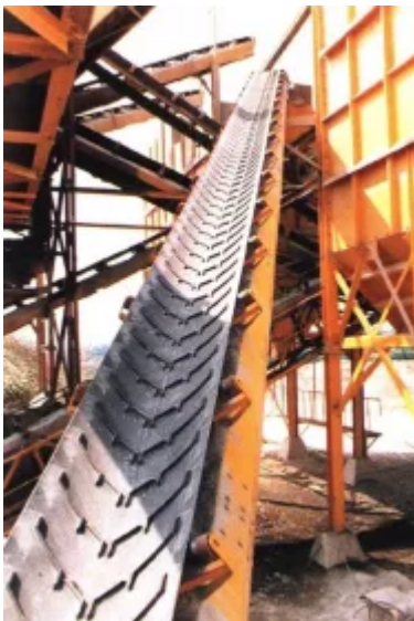
Fig. 8: Unfortunately, Conveyor belts used on mobile equipment are viewed by a great many as readily disposable components.
