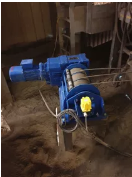
The bespoke electric winch used for the safe and smooth lifting and lowering of a large telescopic export chute.
